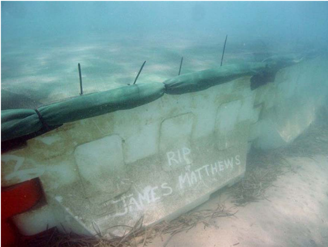
Fig. 6. Shade cloth cover over the top of the cofferdam surrounding James Matthews (J. Carpenter).
